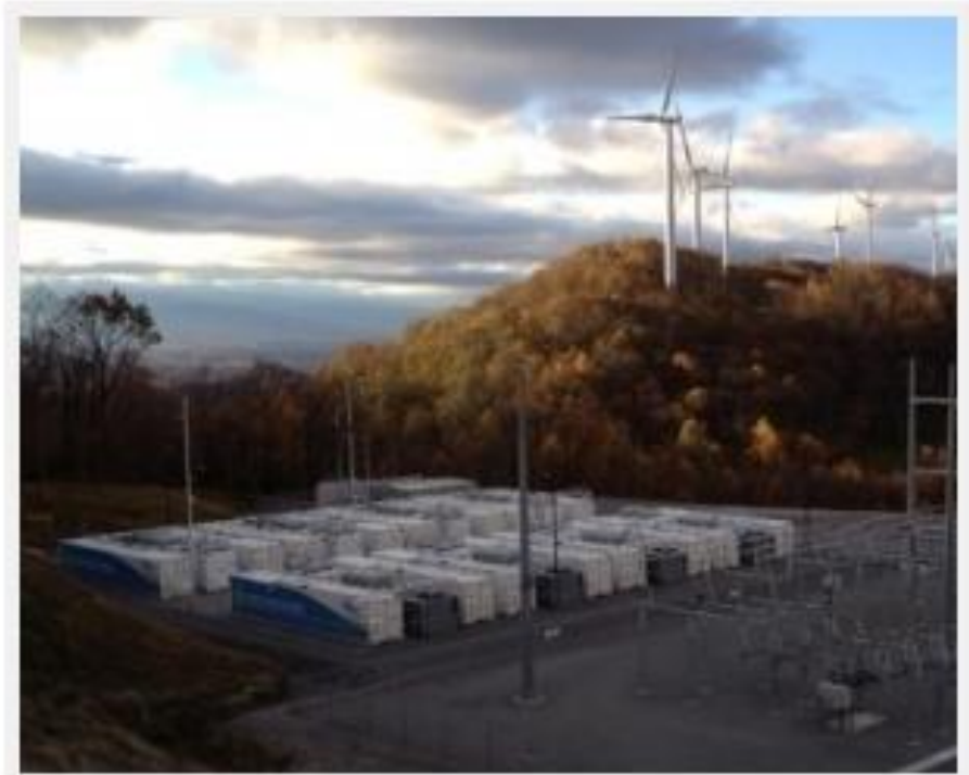
AES's wind and energy storage project in West Virginia
